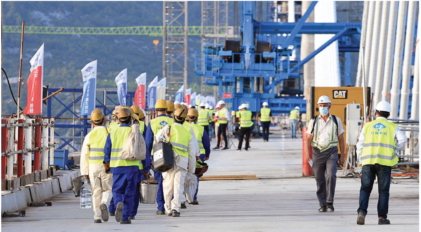
Engineers walk toward the Pelješac Bridge on Croatia's Adriatic Sea coast in 2021. The European Union-funded bridge, built by China Road and Bridge Corp., connects sections of the Croatian coastline divided by Bosnia-Herzegovina. AFP/GETTY IMAGES
